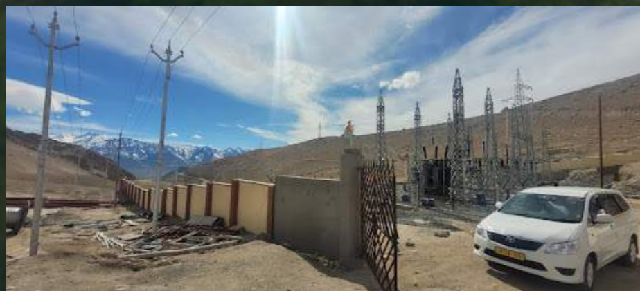
Figure 20: Substation identified near Lungmar area to setup green hydrogen unit
