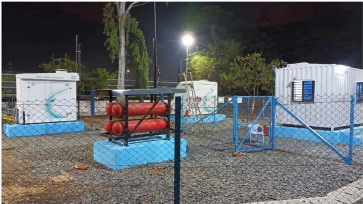
(NTPC Kawas Green H2 Blending project having electrolyser, hydrogen storage and blending skid)
