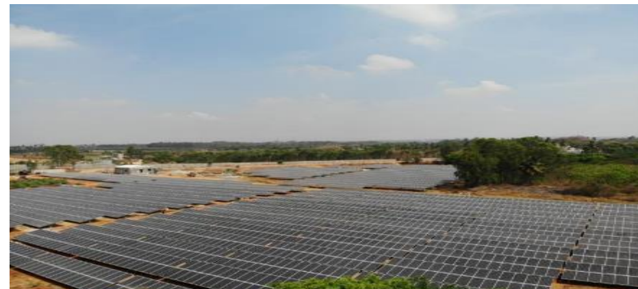
Solar Panels at HRGRDC, Bengaluru
