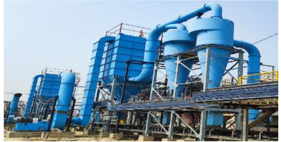
CBG Plant at Budaun- Milling Section
