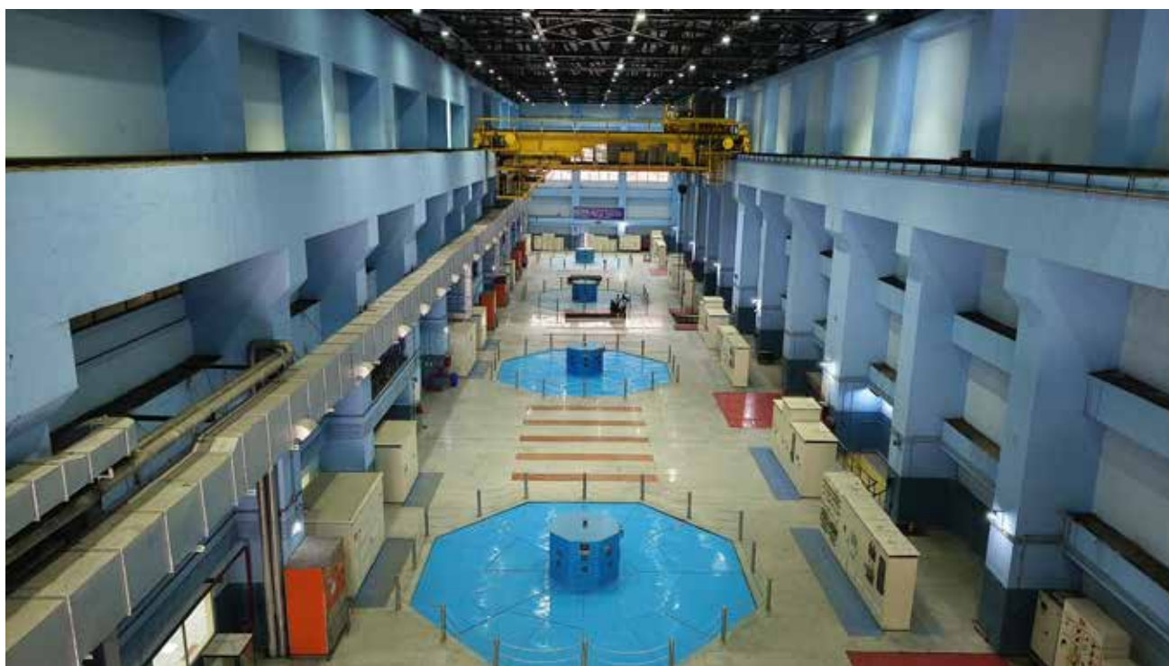
SURFACE POWER HOUSE– 800 MW PARBATI-II (HIMACHAL PRADESH)
